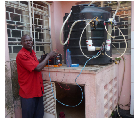
Above: Our water chlorination- saves lives
